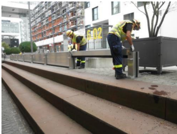
Placing the horizontal beams. Note that the lowest beam is supplied with foam rubber (5 cm thick)
