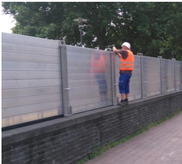
Manually turning the bolts to press the horizontal beams. Note the thickness of the foam rubber.
