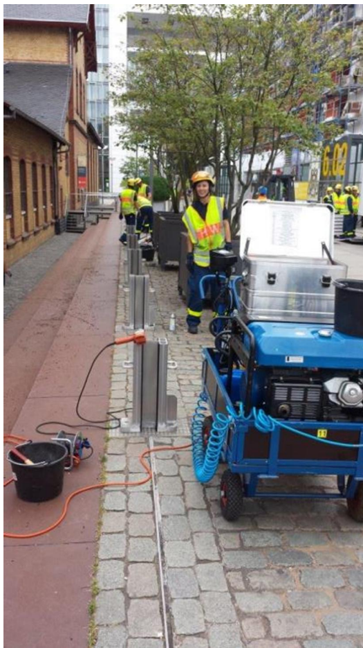
The carts with fixing tools, small generator and other equipment to be used (supplied by Steb)
