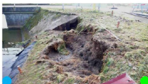
Figure 1.3.6. Ol.3 N = 1260 detail damage
