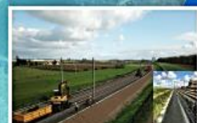
Construction of an inspection pathway over 46 km alongside railway track Hoekse Lijn.
