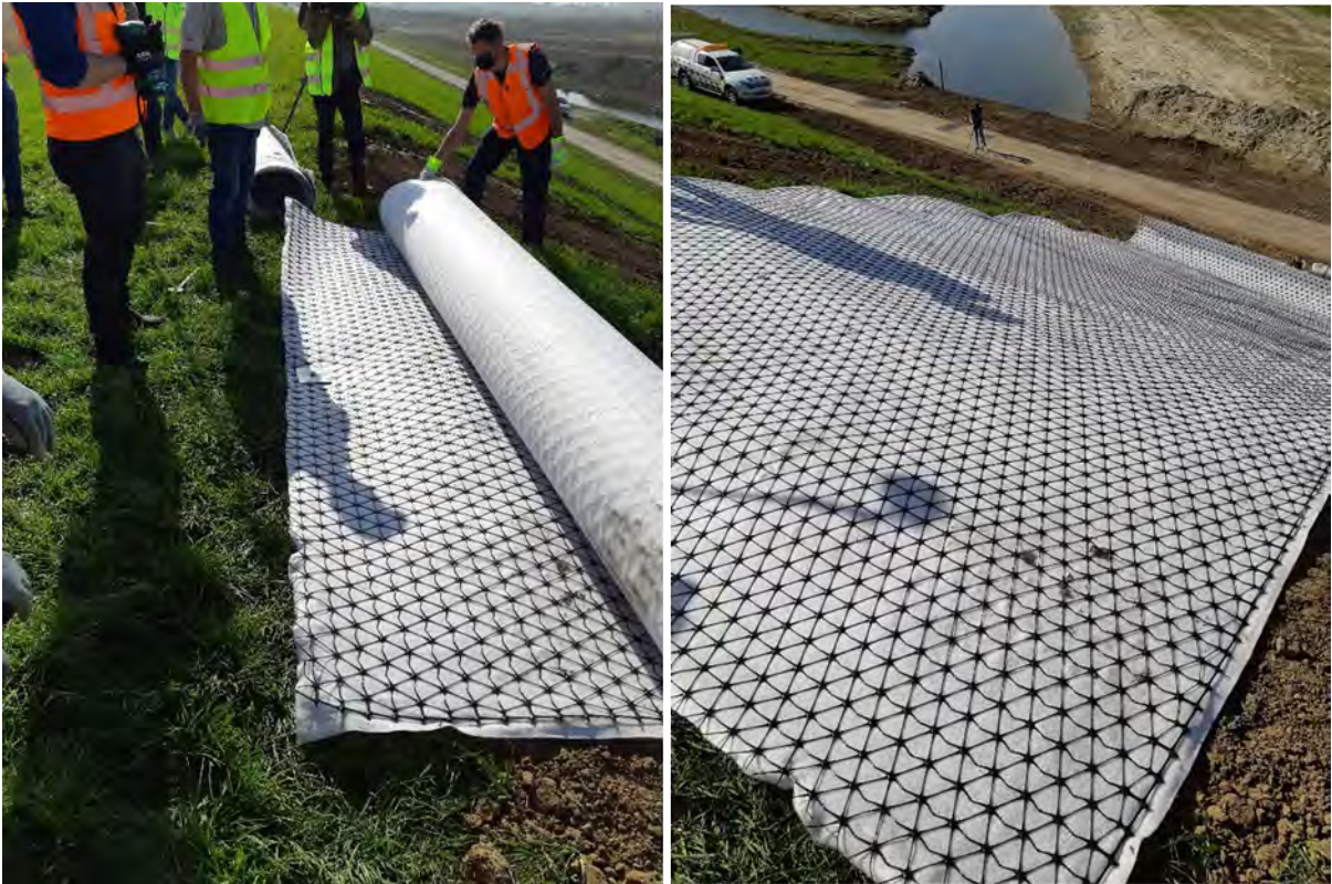
Figure 2.3 Placing of a Tensar panel. The panel is fixed by one Wurmi peg at the crown of the dike before uncoiling it.
