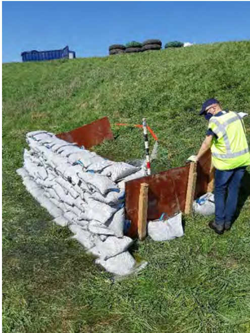
Figure 1.6 The construction was leaking intensively
