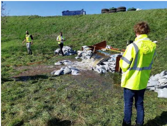
Figure 1.9 Failure of the dam and overflow
