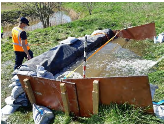
Figure 1.7 Sandbag dam with extra EPDM sheet on the upstream side
