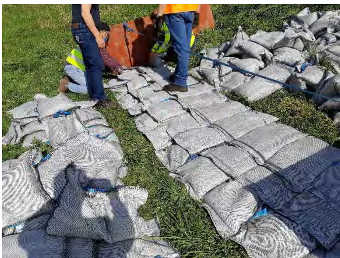
Figure 1.3 The second layer was not placed in a staggered way
