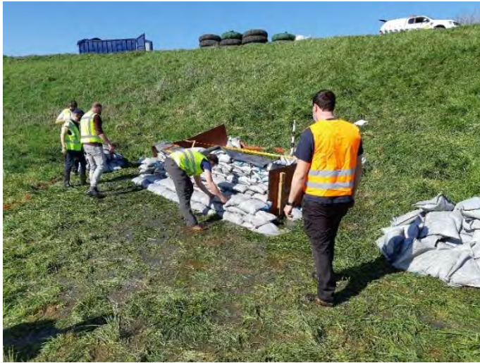
Figure Error! No text of specified style in document..8 Removing sandbags from the outer side of the dam
