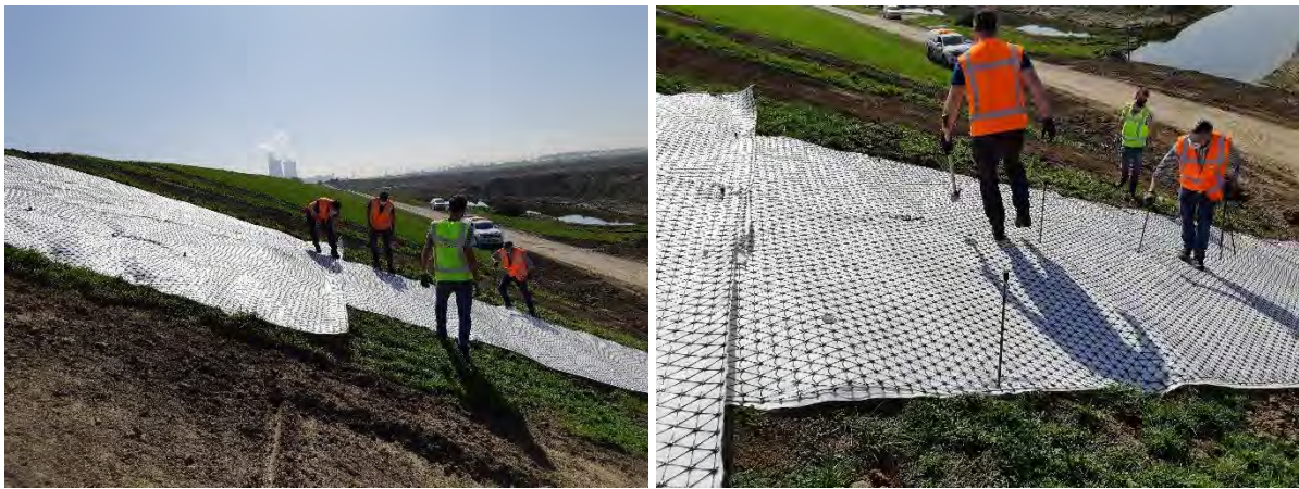
Figure 2.10 Creating an overlap with the third panel. The lower panel is fixed with only one type of pins (Y-pin). A part of the panel is covering the sod of the slope, the main part of the panel is covering the recently sown clay layer.
