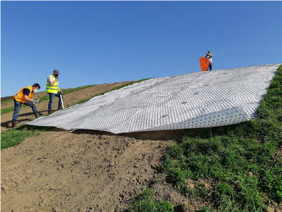
Figure 2.7 The lower part of the panel is not yet fixed, so that the overlap with the following panel can be realized.
