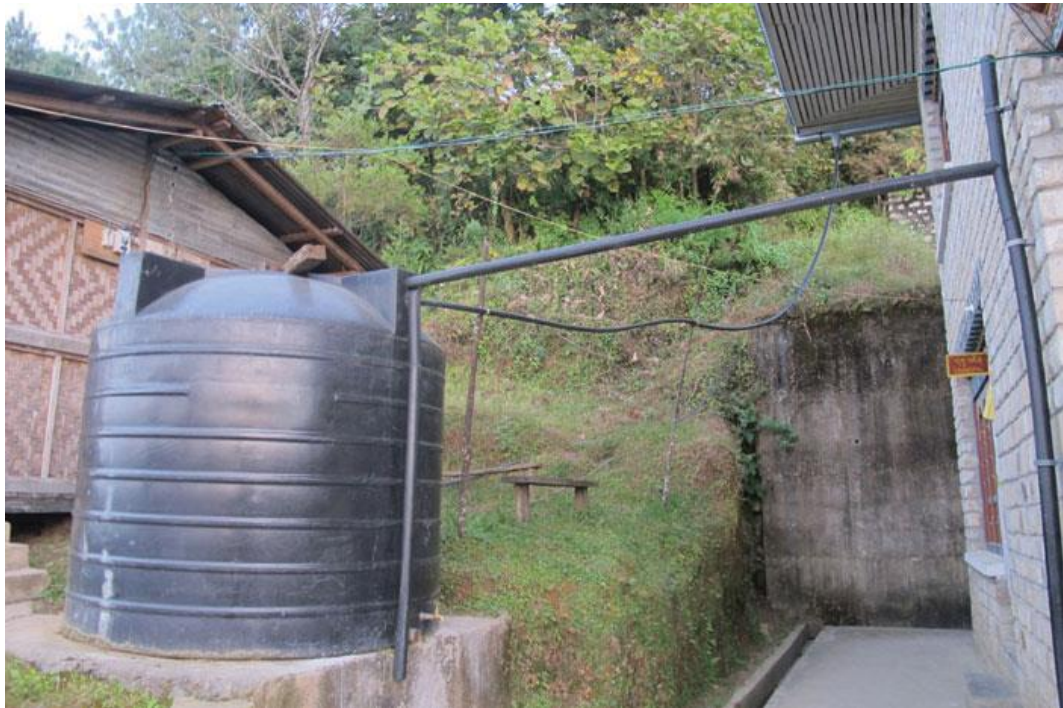
Figure 3-15 Example of a water storage tank linked to the roofs to store rainwater in Bhutan.
