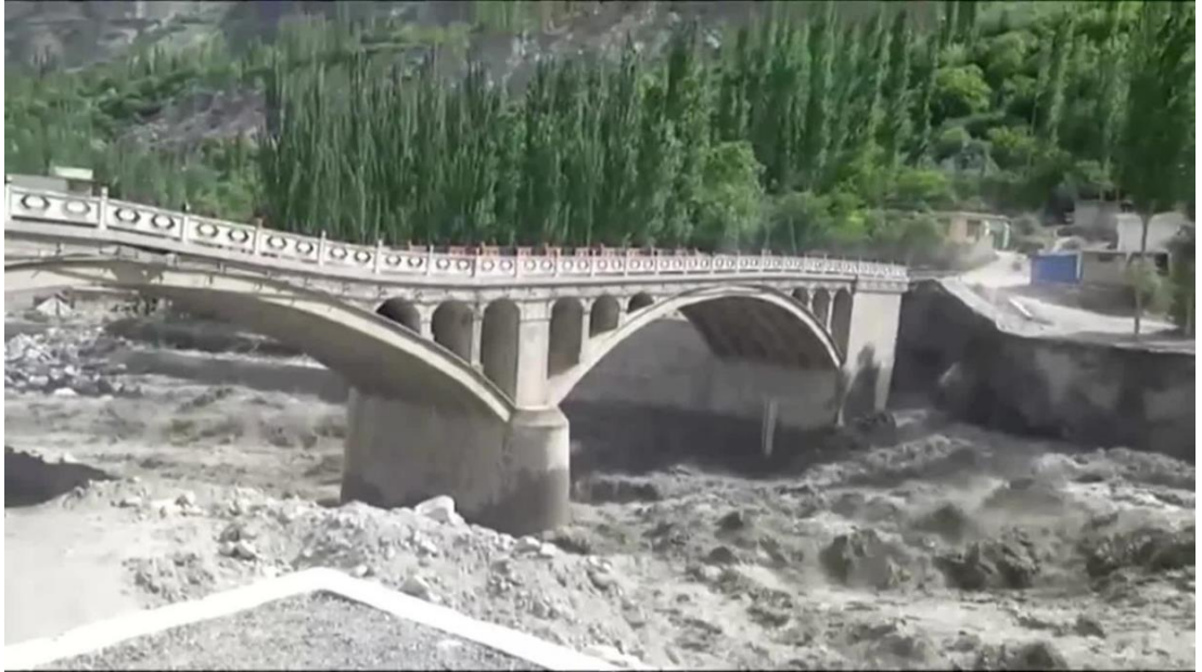
Figure 2-10 Bridge collapse in Pakistan after a glacier lake outburst flood (GLOF) in the summer of 2022. (source: https://www.onenewspage.com/video/20220508/14658895/Pakistan-bridge-swept-away-by-glacier-lake-outburst.htm ).
