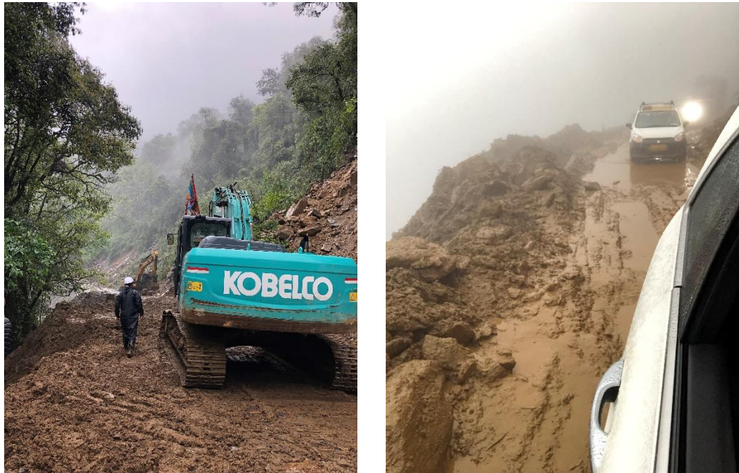
Figure 2-8 Clearance of a landslide (left) and travel conditions after clearance (right) on the road between Sengor and Mongar during the field visit of May 2022.
