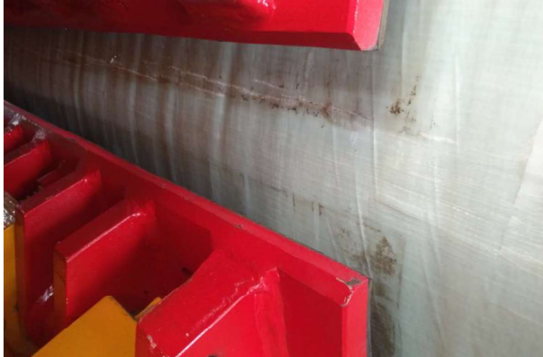
Figure 23: Break of pipe between clamps
