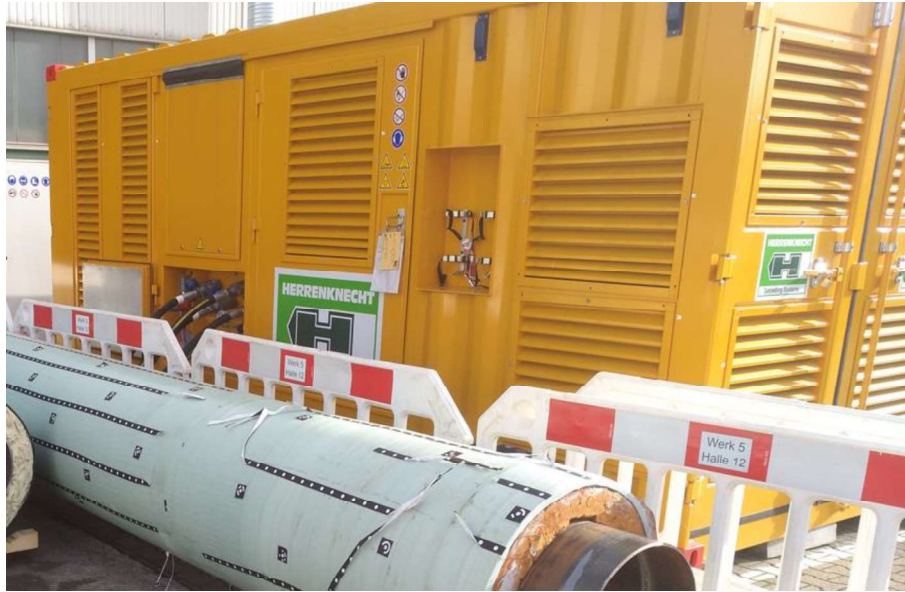
Figure 7: Hydraulic power unit
