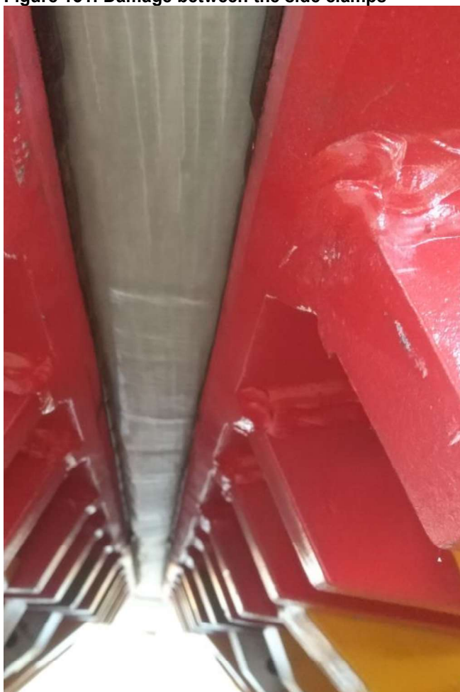
Figure 132: Damage of the pipe between the lower clamps
