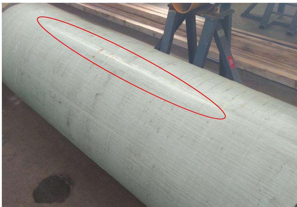
Figure 135: Damaged pipe after disassembly
