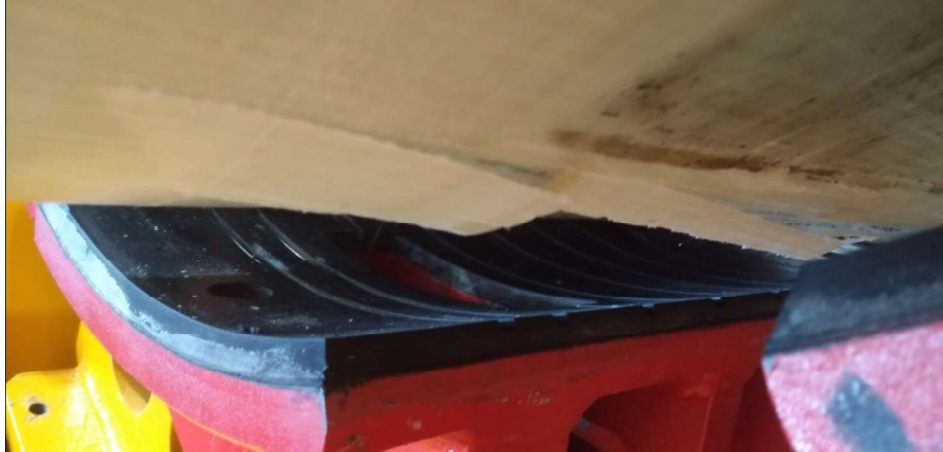
Figure 69: Side view of damaged pipe between the lower clamps
