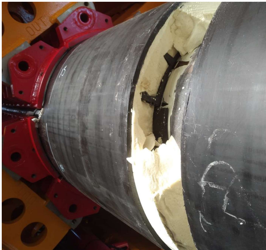
Figure 94: Broken spacer and PUR
