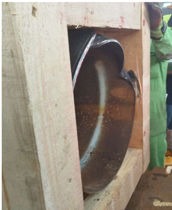
Figure 166: Damaged steel pipe
