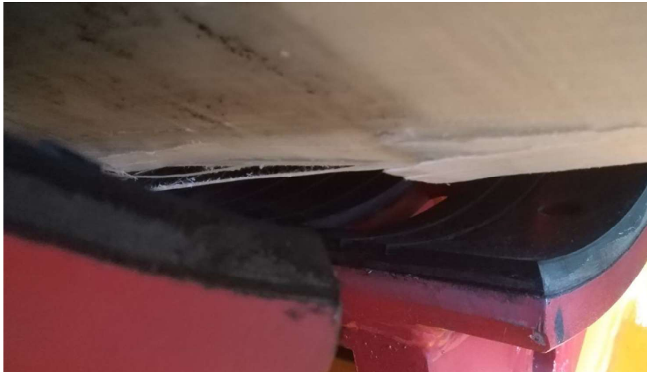
Figure 70: Side view of damaged pipe between the lower clamps
