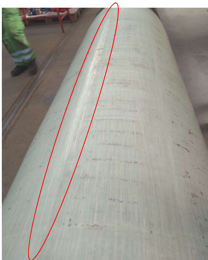
Figure 134: Damaged pipe after disassembly
