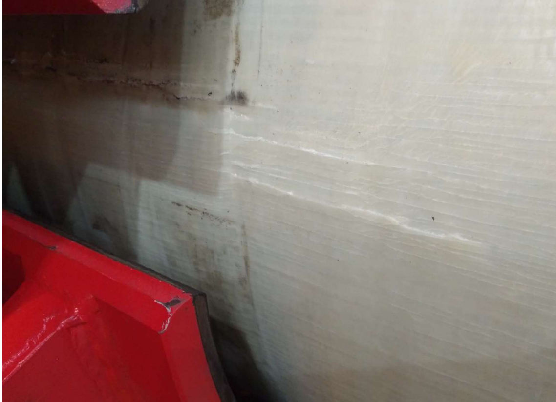
Figure 15: Break of pipe between clamps
