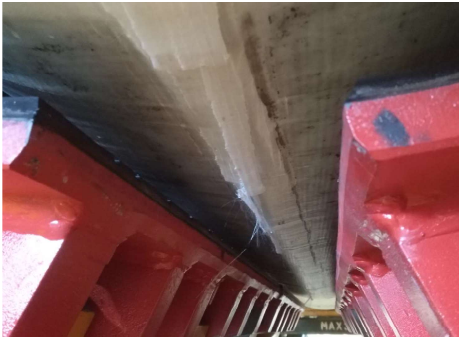
Figure 68: Zoomed damaged pipe between the lower clamps
