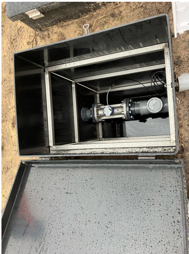
Figure 27 New monitoring station for road runoff along highway A58 near Kloosters.
