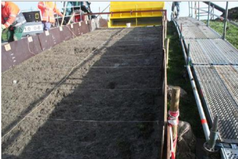
Figure 3.17 Bare clay surface after a few small waves, showing a depression in the middle of the slope and a few small erosion pits (Akkerman et al., 2007).
