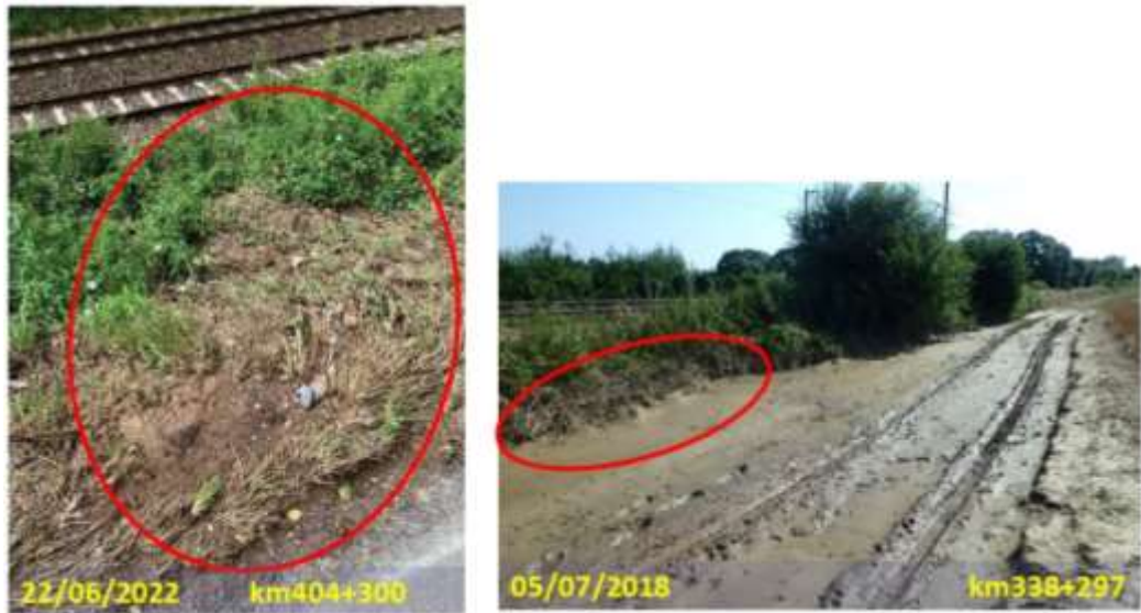
Figure 9 - Photos of incidents on a stretch of track 42000 along the Villaine, near the study area.
