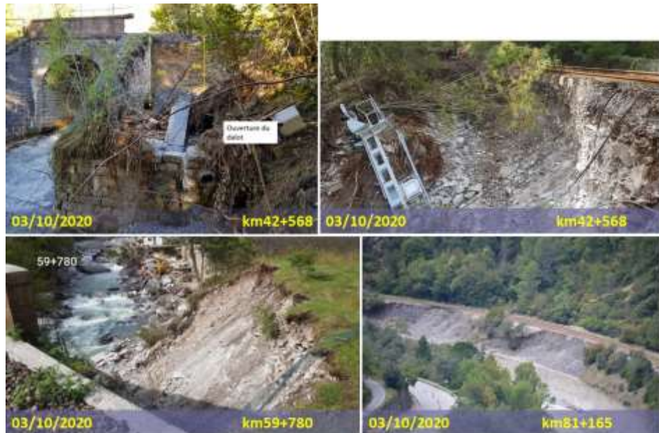
Figure 11 - Images of damages to line 968000 in the Roya catchment due to storm Alex.
