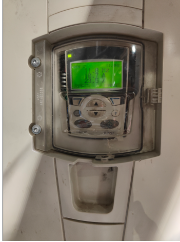
Figure 22: Control panel of pump
