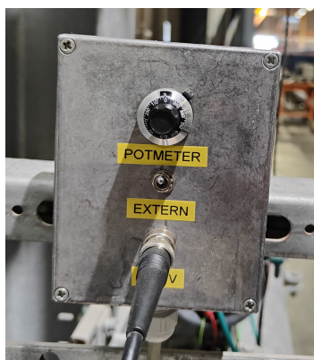
Figure 20: Pump control: Potentiometer
