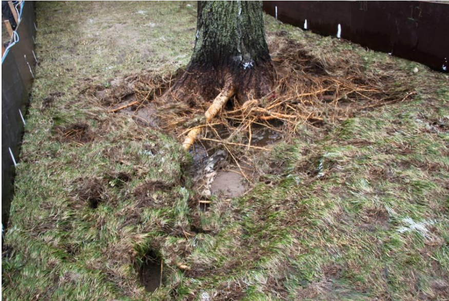
Figure A.2 Erosion at tree; width of test section is 4 m
