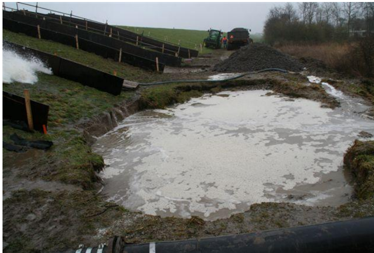
Figure A8 Scour hole at the toe of the dike; sub soil consists of gravel (Kattendijke)
