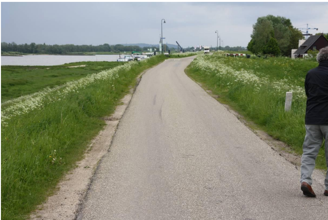
Photo 2.10 Road on the crest, damage is severe close to the asphalt (Location 5)
