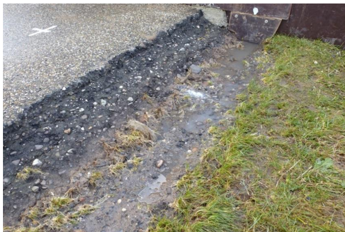
Figure 4.26a Less damage at transition from asphalt road to grass revetment (after 6 h at the end of q = 1 l/s per m)
