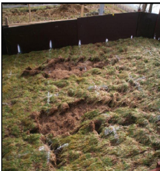
Damage at various locations or multiple open spots
