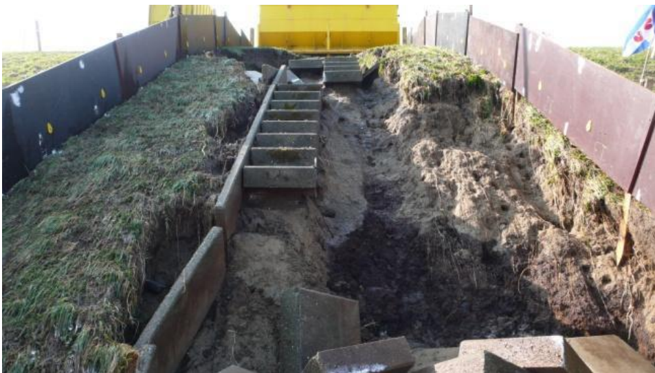
Figure 4.32 Erosion close to stairs (Tholen)
