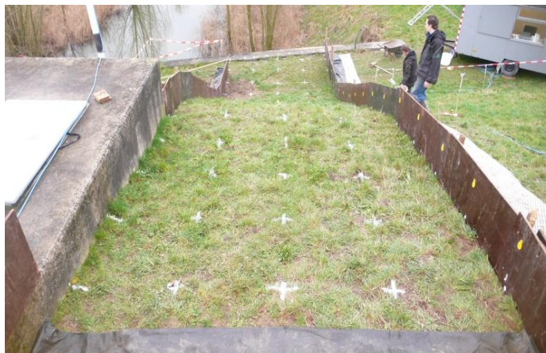
Figure 2.6 Reduction of grass strength along concrete wall (on the left side)
