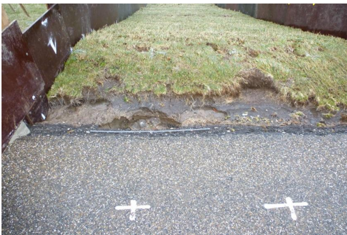
Figure 4.26c Failure of transition from asphalt road to grass revetment (after 14 h or after 2 h with q = 50 l/s per m)
