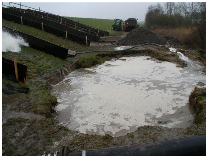
Figure 4.27c Scour hole at the toe of the dike; sub soil consists of gravel (Kattendijke)
