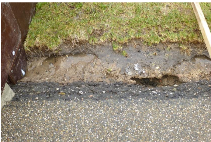
Figure 4.26b Multiple open spots at transition from asphalt road to grass revetment (after 12 h at the end of q = 10 l/s per m)
