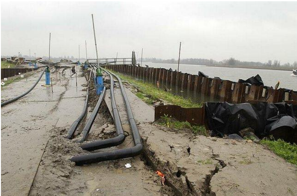
Figure 6.5 Experimental set up: 50 m sheet pile basin (right hand side) was filled to overflow the deformed crest after a slip failure (left hand side)
