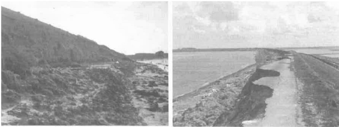
Figure 1.1 Residual dike profiles after wave overtopping induced shallow slip failures after the storm surge disaster of 1953 (Knoeff et al. 2002)
