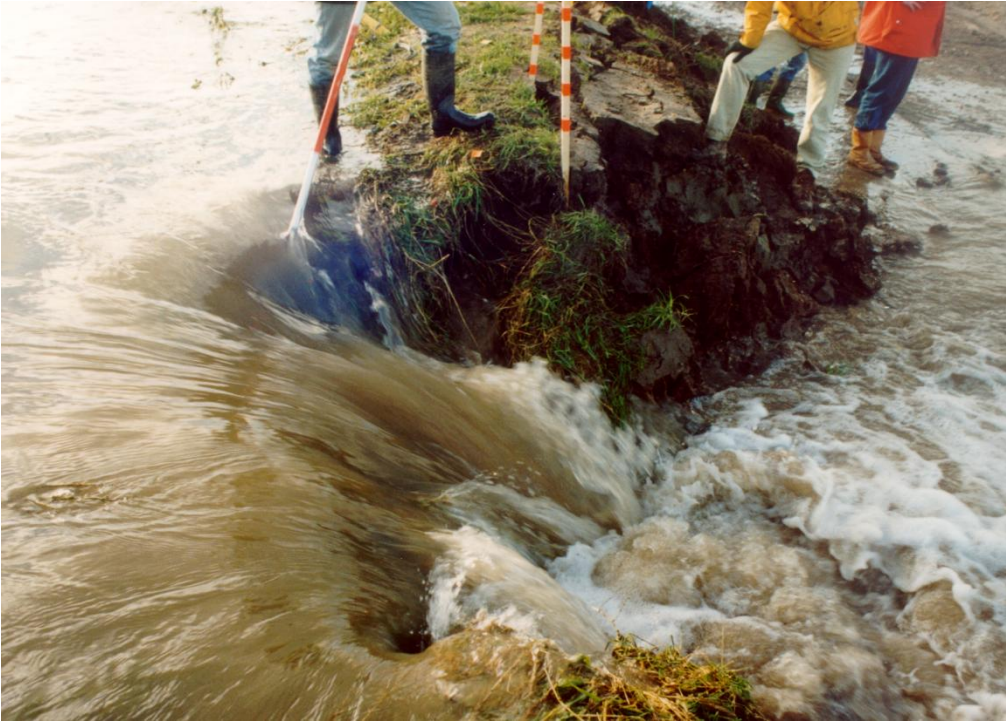
Figure 6.10 Close up of the head cut. The man in the yellow coat stands approximately at the original scarp location
