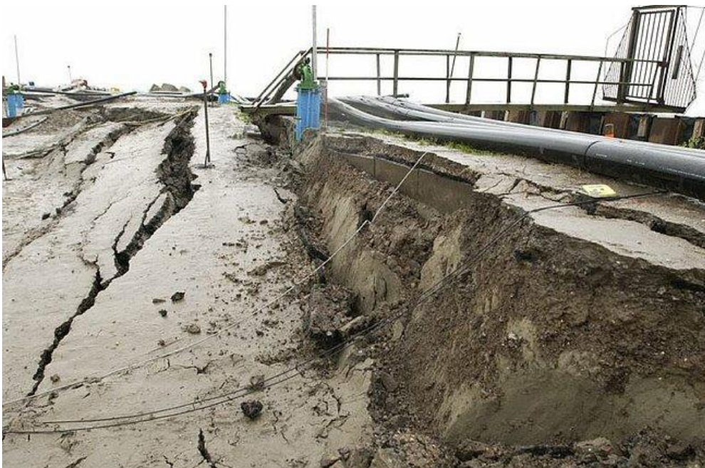
Figure 6.6 Detail of the scarp to be overflowed. Some remains of asphalt and or pavement elements founded on cemented sand and clay
