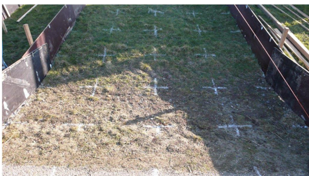
Figure 5.9. Quality of the grass berm was bad at Tholen (before testing)
