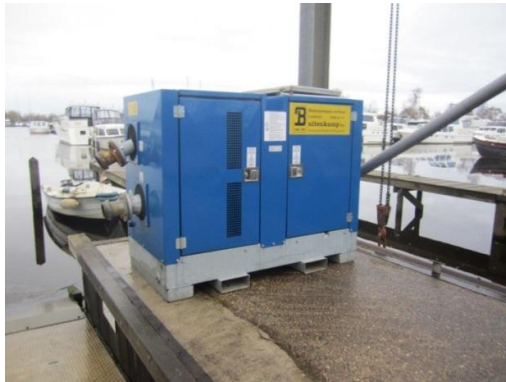
Picture 34. Pump for testing with 7 m
