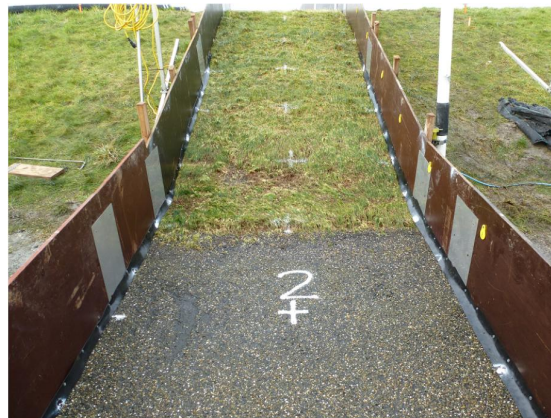
Figure 5.4. Slight erosion at the transition to the upper slope, test 2
