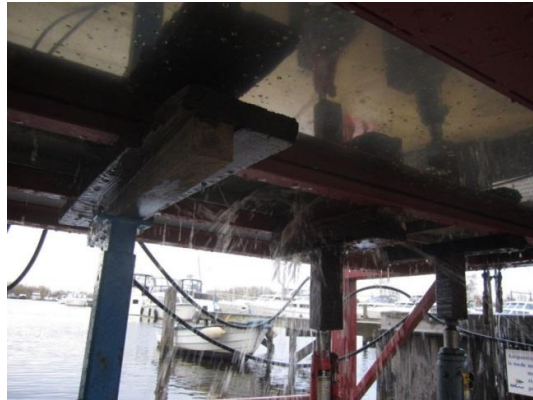
Picture 28. Small leakage with low filling level
