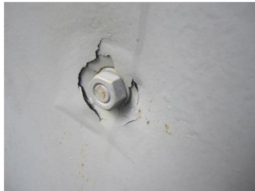
Picture 37. Broken epoxy paint by bending
