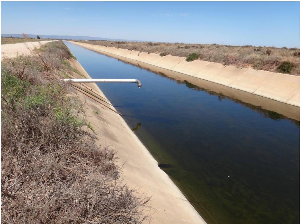
Discharge Channel of Bolivar Wastewater Treatment Plant – Photograph by SA Water
