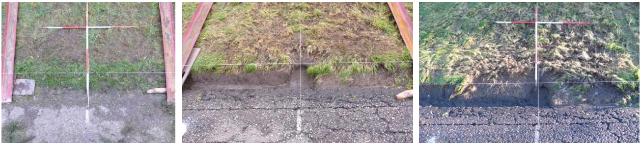
Figure 13. Impression of Test Section Ha.3 (horizontal transition from asphalt to grass). Left: initial condition. Middle: condition prior to impact 1360 with artificial damage including a gutter. Right: impression of damage after a total of 2360 impacts.
