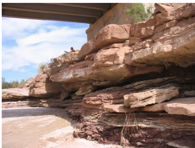
Scour in rock (sandstone; HEC 18)
