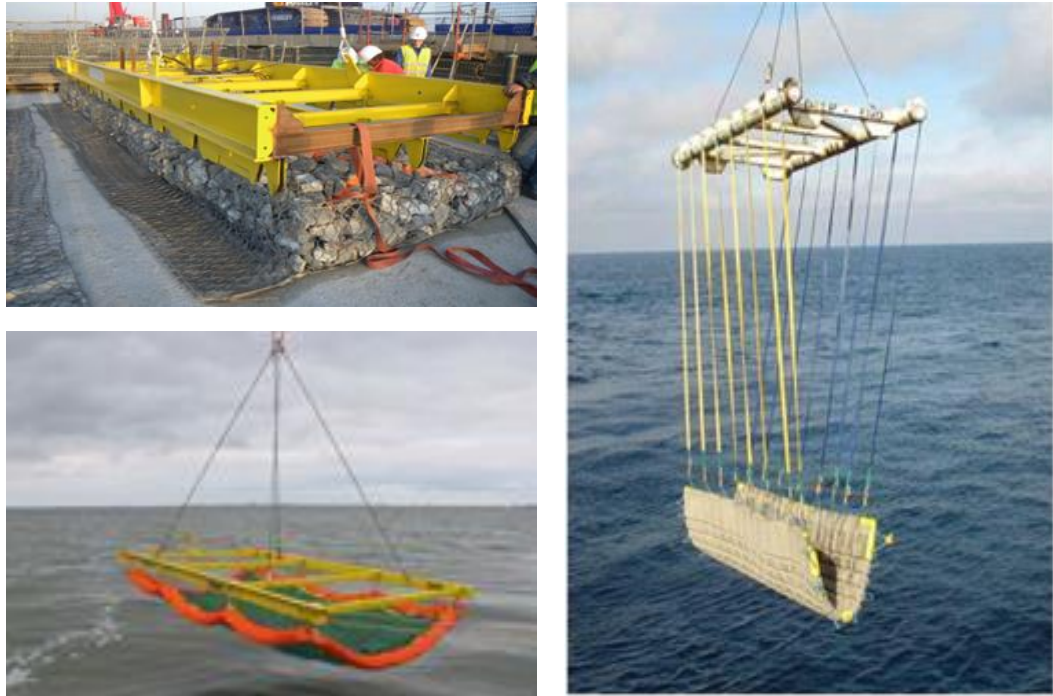
Figure 9.3 Examples of lifting arrangements with different alternative systems. Top left: automatic lifting frame for gabion mattresses. Bottom left: lifting of frond mat. Right: concrete mattress suspended by 16x 6 m webbing slings.
