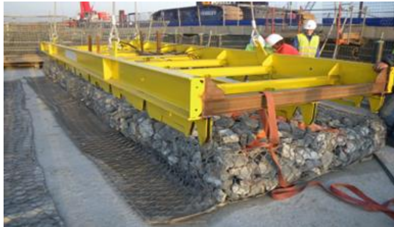
Figure 11.27 Installation of a gabion mattress with side bands using an automatic frame.
