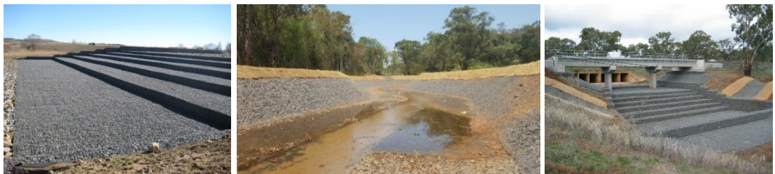
Figure 11.2 Examples of gabion mattress functions ( www.maccaferri.com ): stepped weir (left), river bank protection (middle) or scour protection at a bridge(right).
