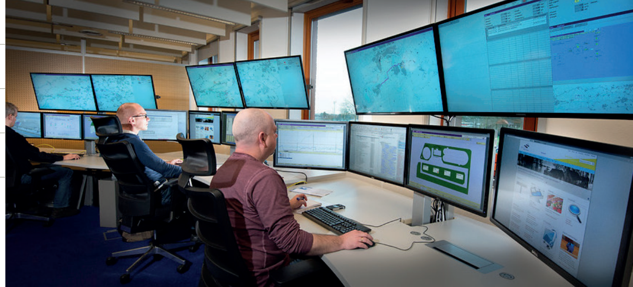
Control room of the Rivierenland water authority, a participant in the JIP Slim Malen (source: Rivierenland water authority)
