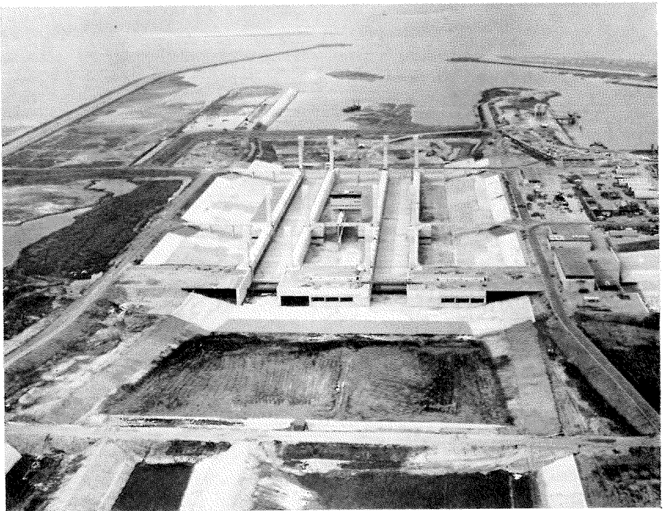
Photo 13. General view of the Kreekrak lock system just before the flooding of the construction site. The concrete work has been completed. The forebays are being dredged to the requisite depth.
