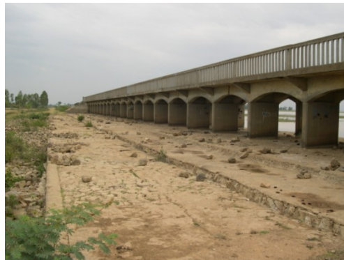
Figure 6: Example of scour protection of the bottom downstream the bridge.
