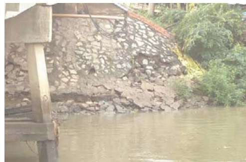
Figure 7 Damage to a bridge abutment.
