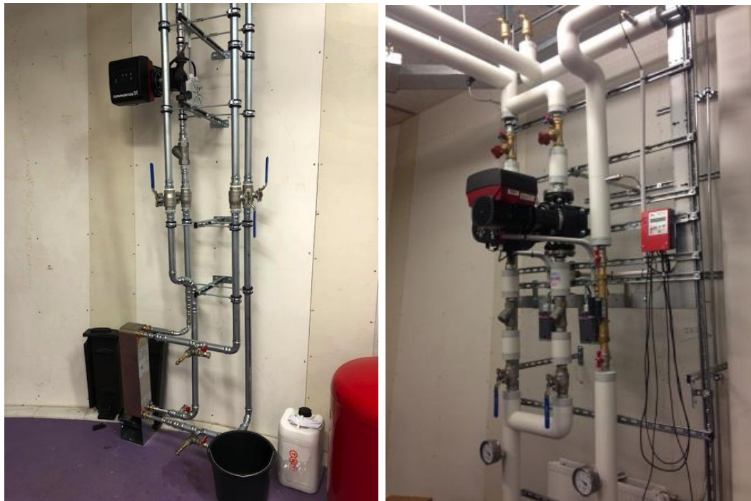
Figure 7. Plant room installation for solar thermal array: heat exchanger (left), array pumping station (right).
