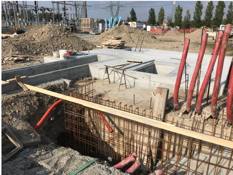
Figure 16. Realization of the technical vane for heat exchange between primary (groundwater) and secondary circuits of the pilot plant.
