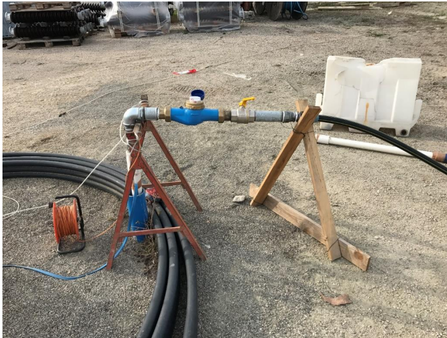
Figure 24. The extraction well with the pump and measuring/regulating devices installed.
