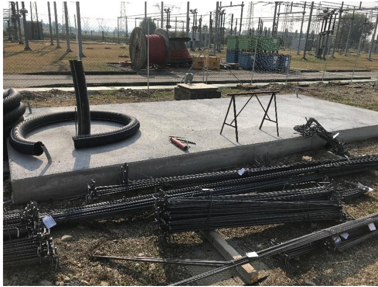
Figure 15. Realization of the technical vane for hydraulic connection of the pilot plant with building A.
