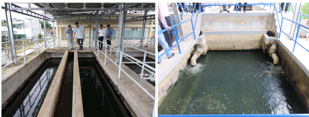
Figure 3: Settling tank (left) and filtration tank (right) at Vi Thanh WTP.
