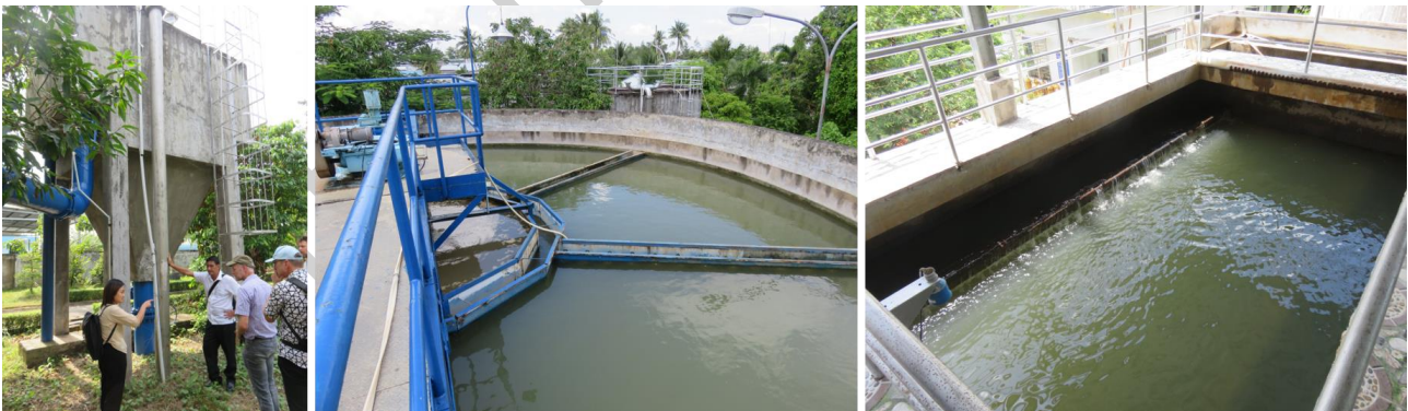
Figure 9: Flocculation tank (left), settling tank (middle) and filtration tank (right) at Nga Bay WTP.
